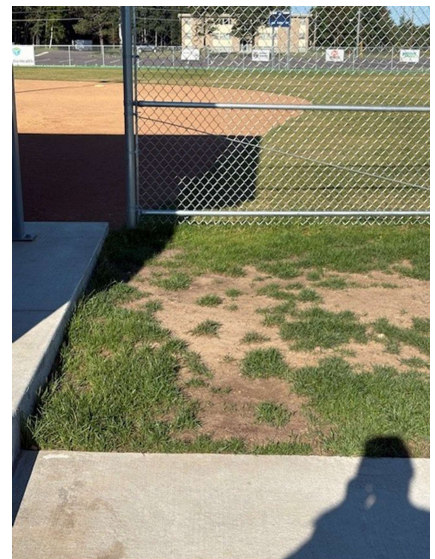
AREA 19 – REPLACE WITH CONCRETE
