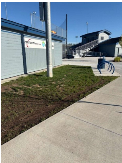
AREA 3 – REPLACE WITH SOD
