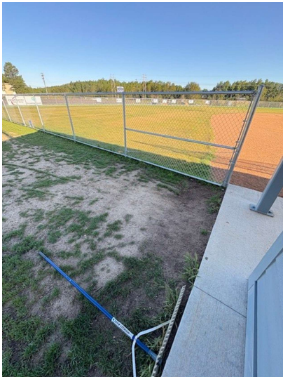
AREA 11 – REPLACE WITH CONCRETE
