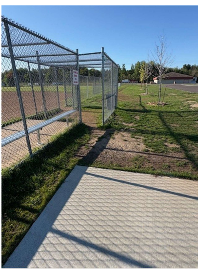
AREA 21 – REPLACE WITH CONCRETE
