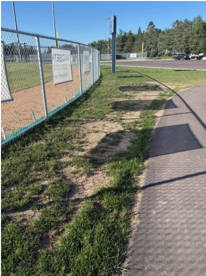
AREA 14 – REPLACE WITH SOD
