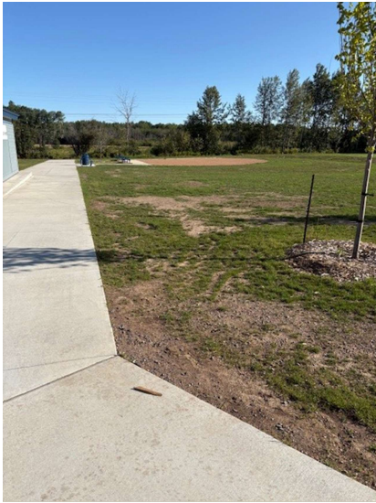
AREA 20 – REPLACE WITH SOD
