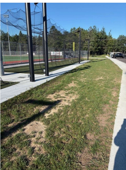
AREA 7 – REPLACE WITH SOD
